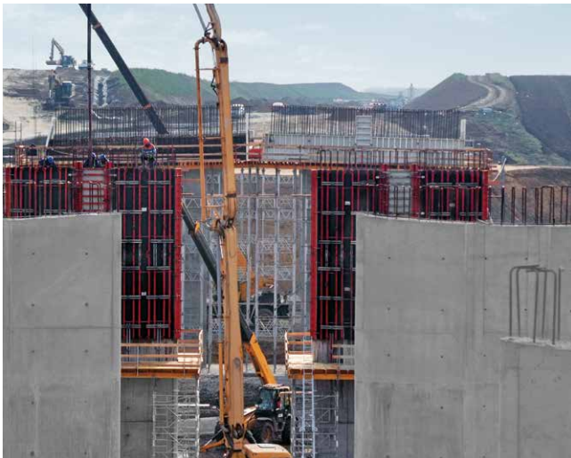
Double bridge piers for a motorway bridge in Bóly, Hungary (standard and special formwork).
