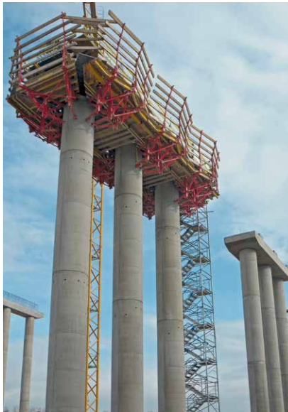
Viaduct over the M6 motorway near Budapest, Hungary (Circo circular column formwork, KLK 230 climbing system).
