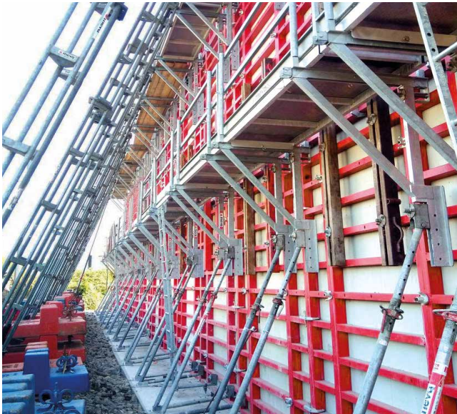
Road bridge over a railway line in Le Versoud, France, with slender set-up of Mammut 350 and SecuritBasic for safe working practices right next to the railway tracks.
