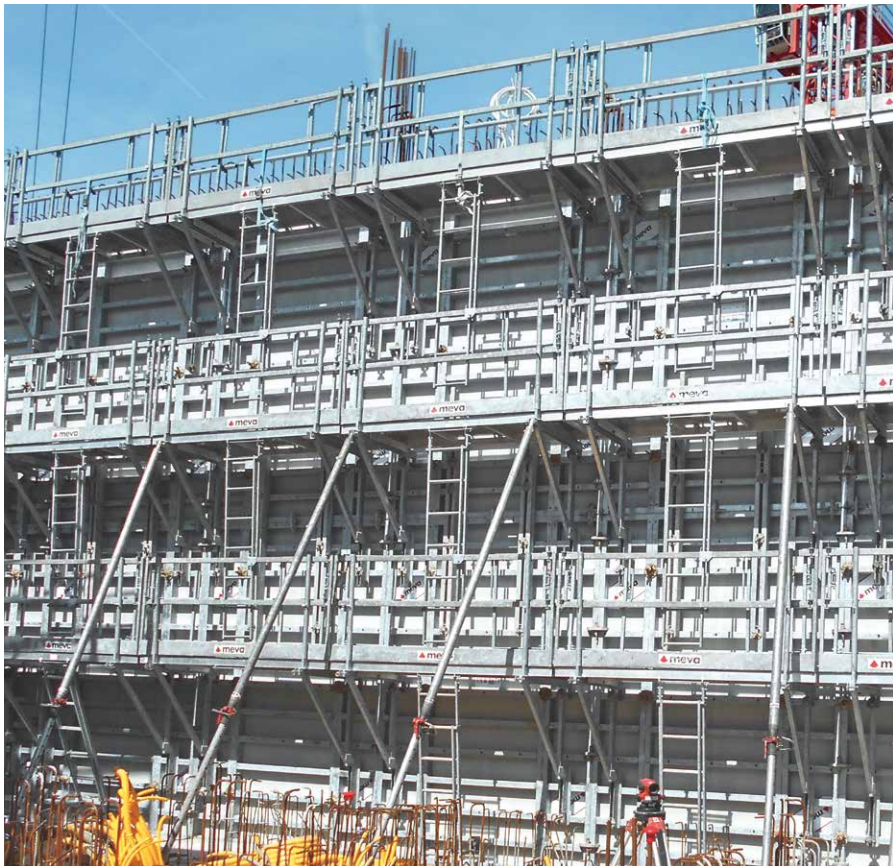
Due to the dimensional accuracy and efficiency of the Mammut 350 formwork, it was possible to pour concrete up to a height of 4 metres without taking the rate of placing into account.
