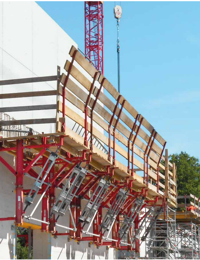
The KLK 230 climbing scaffold was used as a barrier-free working scaffold to enable the formwork to be precisely aligned.
