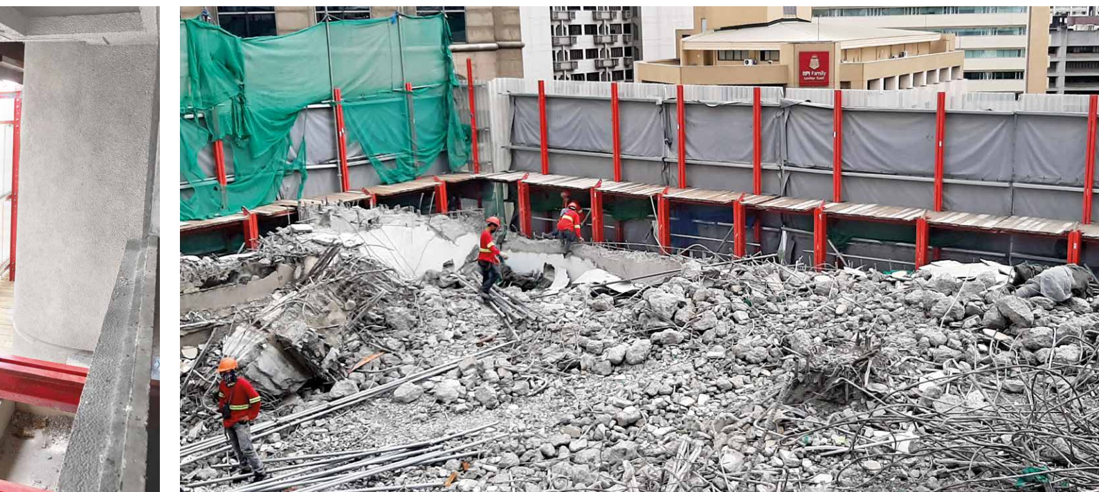
Demolition work on one of the 21 floors: The MGS screen system enabled safe and rapid dismantling and protected the surrounding area.
